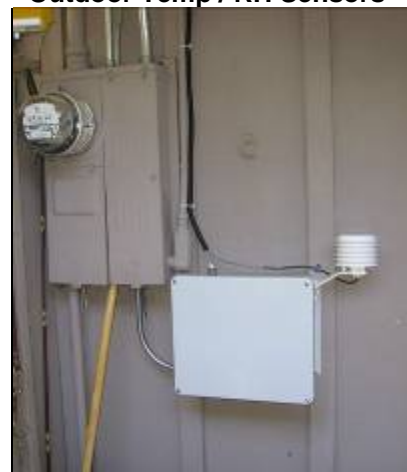
Figure 8. Electricity Use & Outdoor Temp / RH Sensors
