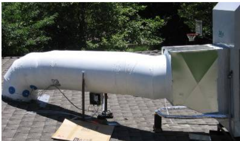
Figure 7. Supply Air Duct Sensors
