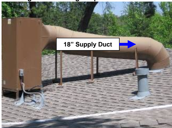
Figure 1. Existing Evaporative Cooler
